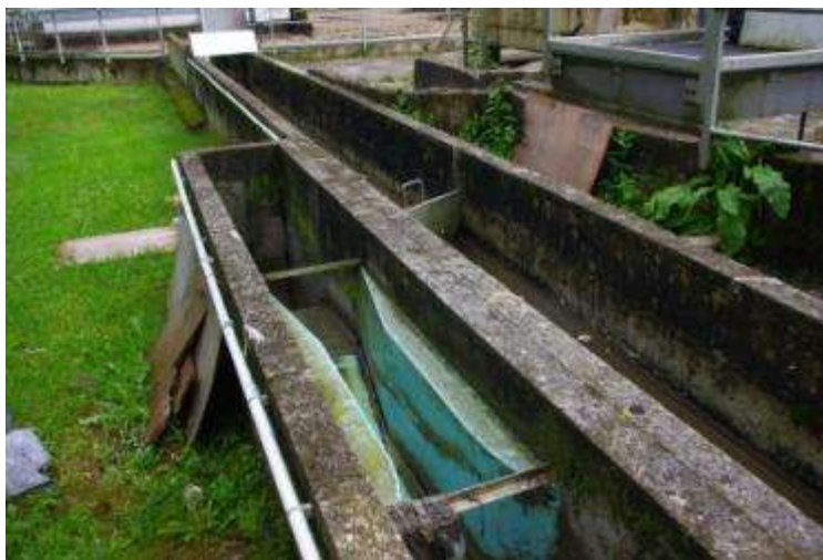
Fig. 16. Canal de by pass
