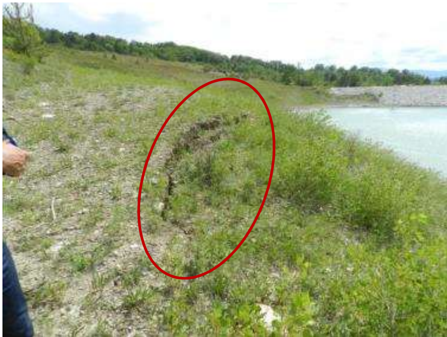
Figure 9 : Fissuration (Source : Irstea)
